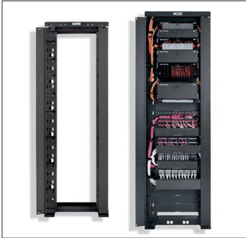
Figure 2 Panduit Distribution Rack
